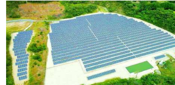
Kanzaki PV Plant
