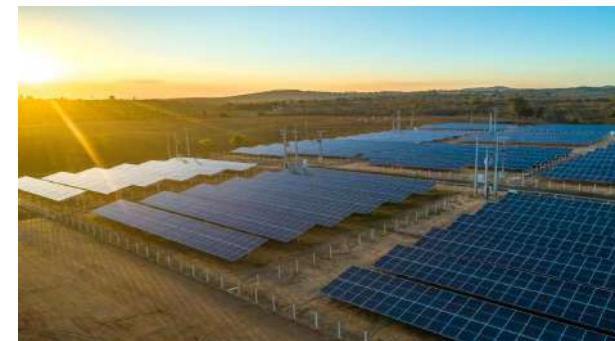
Setta PV Plant
