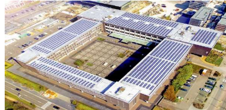
Genk City Hall Rooftop PV Project
