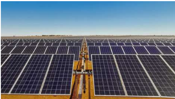
Kimberly Droogfontein PV Plant
