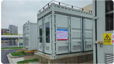
State Grid Sodium-Ion Battery Energy Storage System
